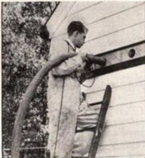
COMPLETELY INSULATED: Our Gimco dealer sent a crew of trained workmen who quickly blew the insulation into our side walls and over the top floor ceiling, too.
